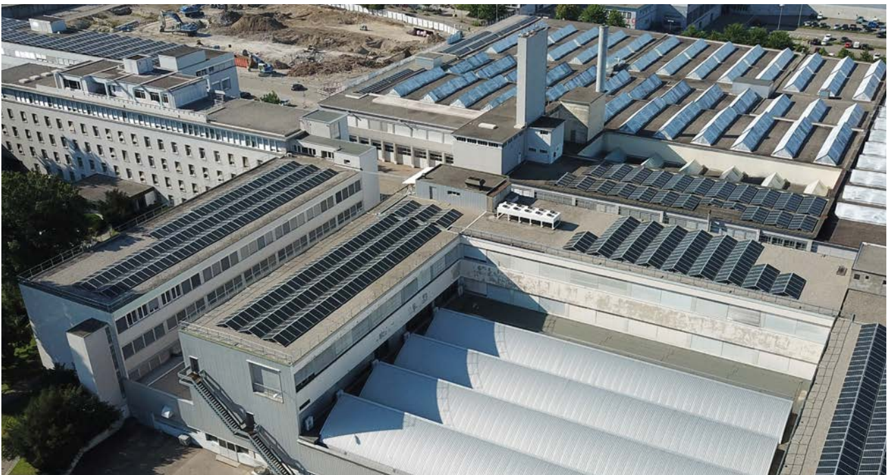
Photovoltaic installation at Rieter Winterthur: The energy mix changed significantly in 2020 compared to the previous year.
