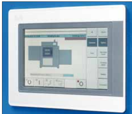
Fig.3 - Touch-screen control panel
